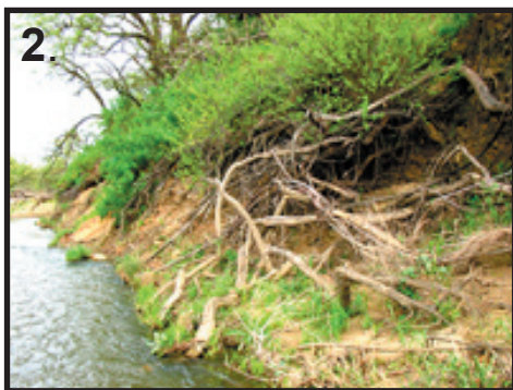
2. Closeup of the section of Putah Creek that was undermining Putah Creek Road.
