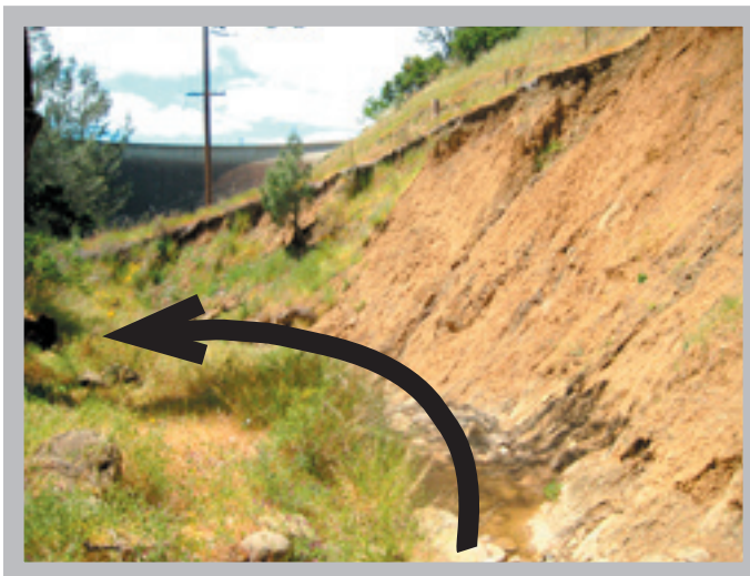
Thompson Creek: Upstream view of eroding bank just above access bridge to Monticello Dam
