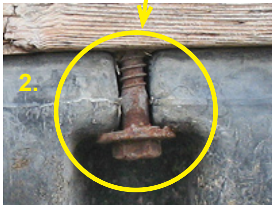
(1). Exposed dock showing ideal area for mussel colonization and monitoring. Early colonization typically takes place in dark, recessed areas such as the bolt grooves shown above. (2) Enlarged and lightened using Photoshop CS3.
