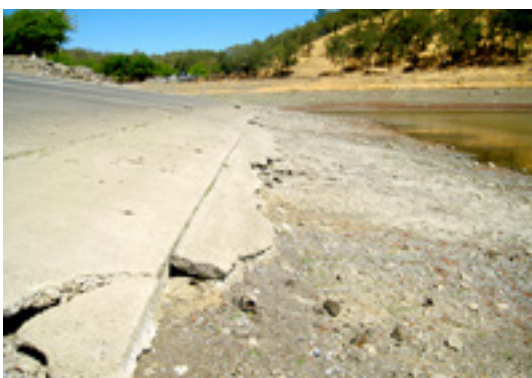
Exposed lower end of launch ramp at Spanish Flat Resort, Lake Berryessa. Site statistically high as a settlement site for mussels.
