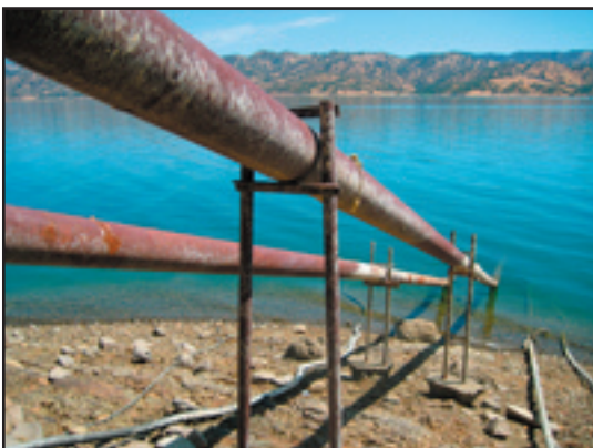
Lake Berryessa. Water intake pipes for Spanish Flat Resort. Pipes and support structure inspected for adult dreissenid mussels.
