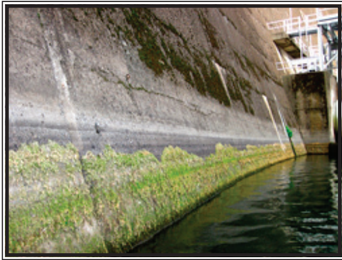
Monticello Dam: Shows algae on dam face.
