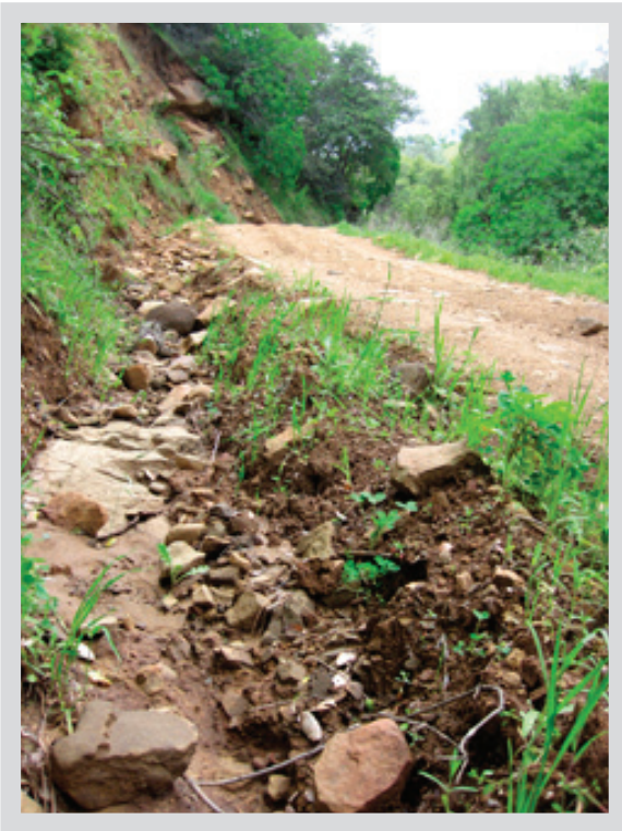
Gully along road into Thompson Canyon.
