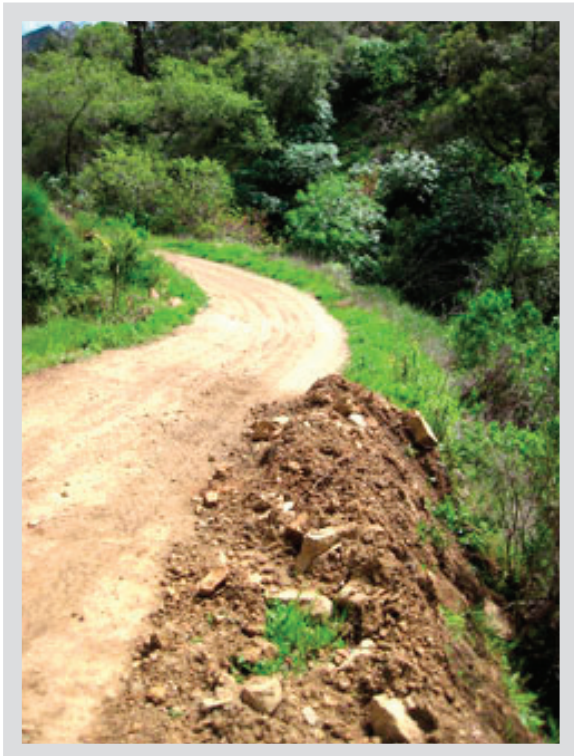
Area with excess materials dumped in creek
