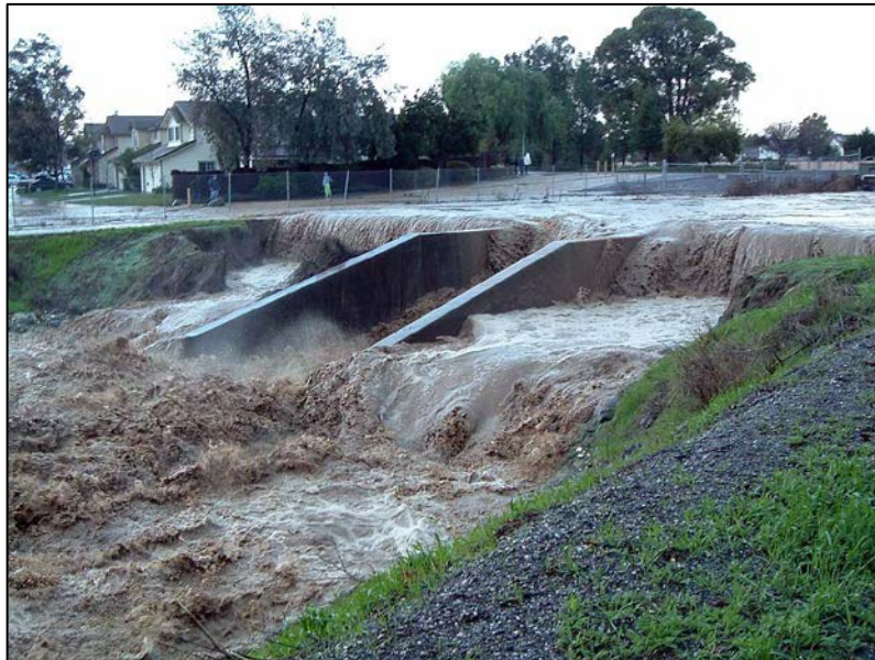
Ulatis Flood Control Channel at Nut Tree Road, Vacaville (Dec 2005) Photo credit: Thomas Pate
