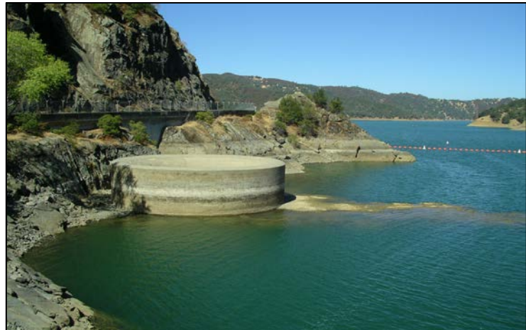
“Glory Hole” Spillway at Lake Berryessa (2008) – 28 ft. diameter Photo credit: Thomas Pate
