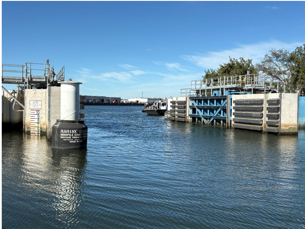
Flood control gates in the Stockton Deep Water Channel. The mussels are now so prolific they prevent the flood control gates from opening and now require manual cleaning by divers on a quarterly basis to function properly.
